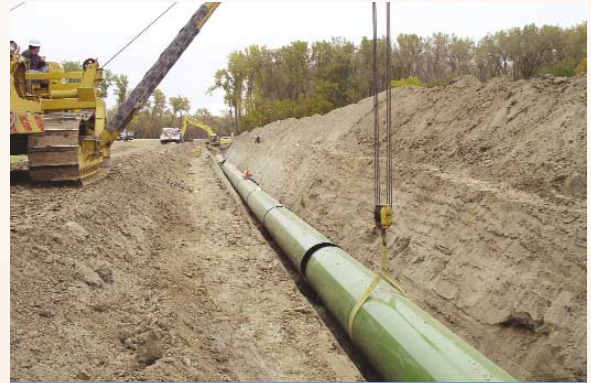
A sideboom crane lowers a 40 foot section of 54" diameter pipe into the 11 foot deep trench on RWP-2.
