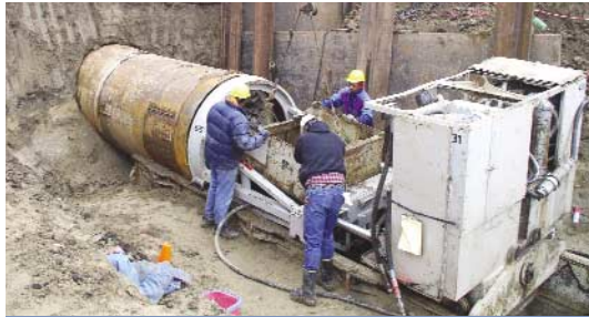
The cart used to excavate the dirt for a boring on RWP-3 is lowered back into place by a crane.
