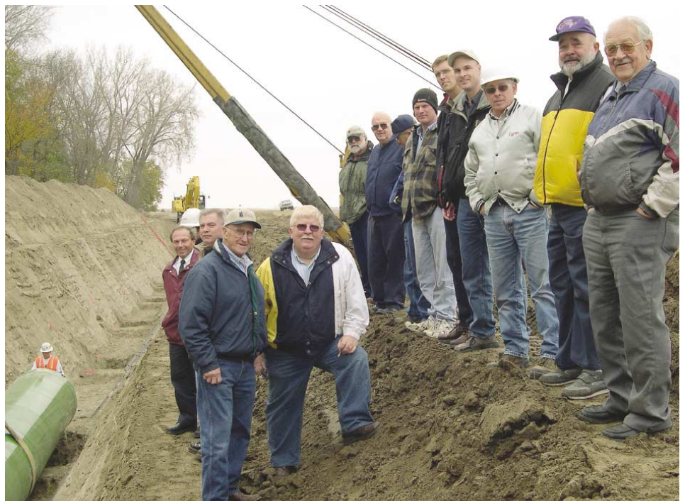
Lewis & Clark directors and officials from the member cities and rural water systems tour the construction on RWP-2 in late October.
