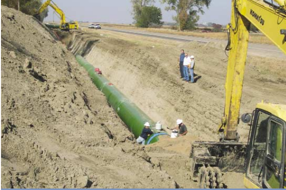
Trench packer waits for a joint to be sealed before packing the bedding material on RWP-2 along Highway 19.
