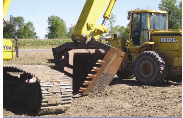
The tapered mining grade bucket, used to excavate the trench on RWP-2, holds 7 1/2 yards of material.
