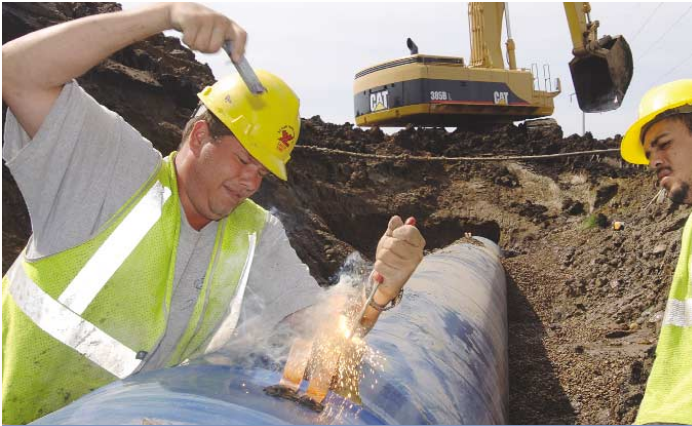
A worker welds a bonding strip to connect two sections of pipe. This will provide electrical continuity for the cathodic protection system.
