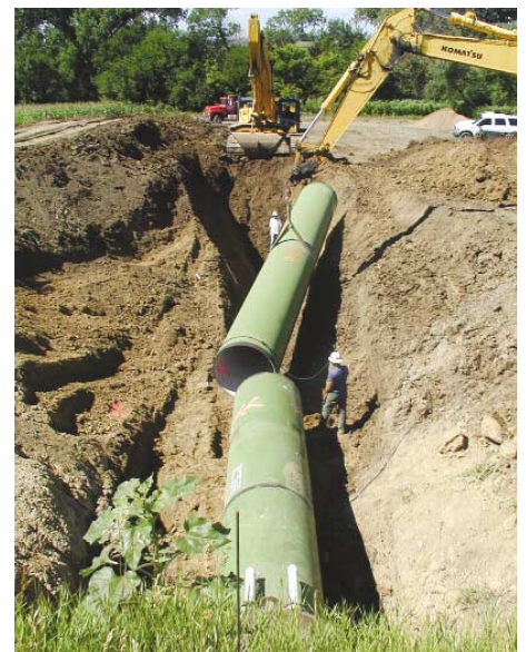
54" diameter pipe section is lined up with another extending from a casing that has been bored under Bluff Road near Vermillion.
