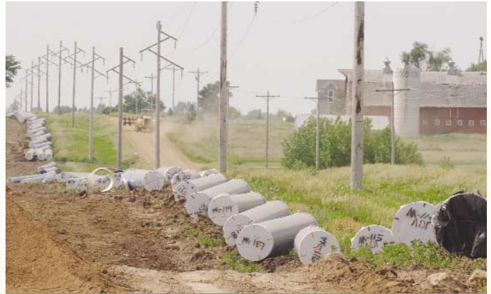
40' long pipe sections lined up along 467th Avenue, two miles west of the Tea-Ellis Road
