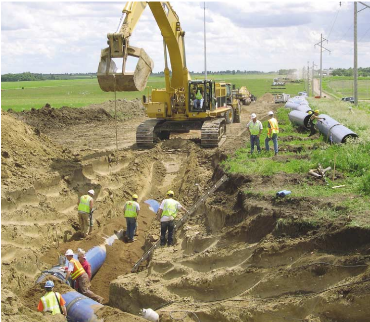
The route for TWP-1 heads south after crossing over from the west side of 467th Avenue to the east. Blue protective coating is used to mark the treated water line and green designates the raw water line.
