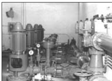
—Inside the treatment plant at South Lincoln Rural Water System
