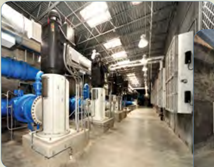
Four 1,250 h.p. motors and pumps in the high-service pump station. There is room to add four more pumps in the future as demand warrants.
