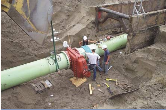
Installation of a 30" diameter gate valve assembly on RWP-1. The valve assemblies will be enclosed in concrete vaults.
