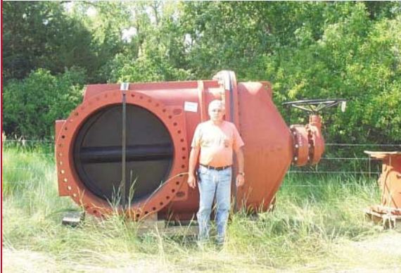
Banner Inspector Lynn Hjellming next to a 48" diameter gate valve that was installed on RWP-1
