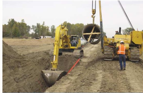
A side boom crane moves a 40 foot long section of 54" pipe on RWP-2. The excavator uses a mining grade bucket that holds 7 1/2 yards of material.
