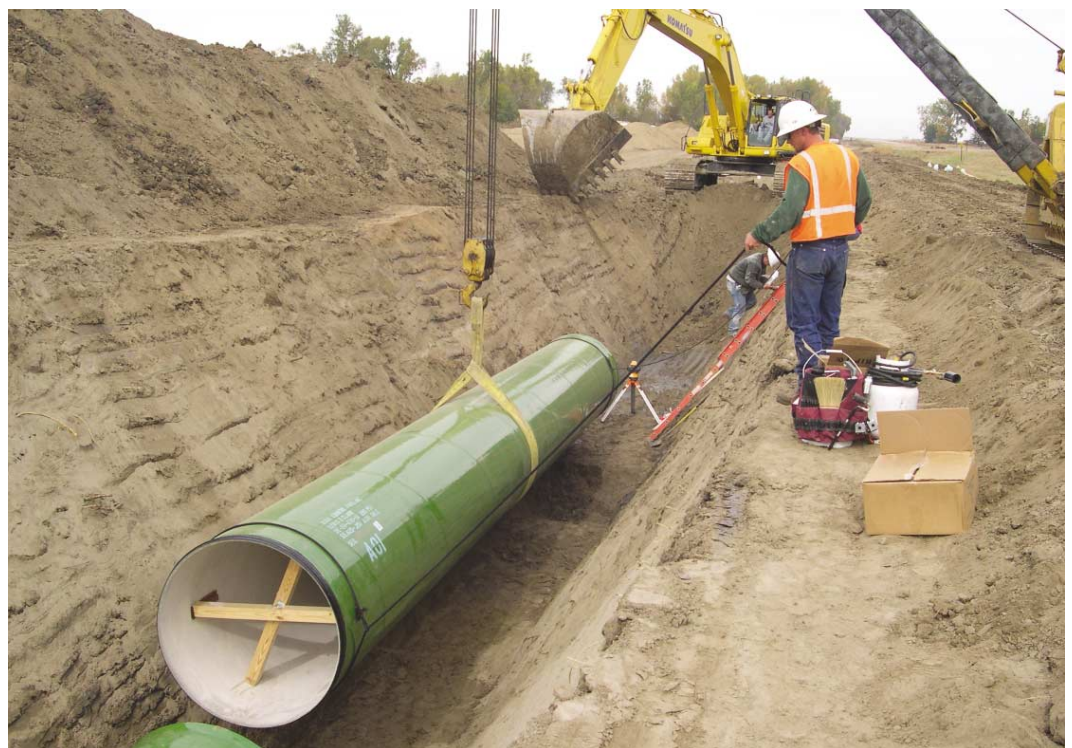
54" diameter steel pipe being lowered into the 11 foot deep trench on RWP-2 along Highway 19
