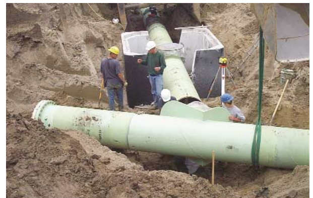
First joint of pipe (30" diameter), with an air release valve vault in the background
