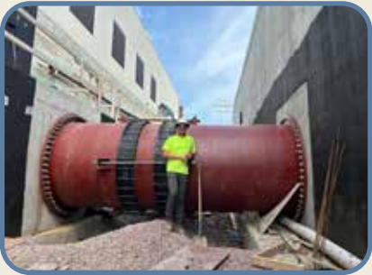
Banner's onsite rep Trevor Stahl next to the 72-inch clearwell effluent pipe that carries treated water from the clearwell to the high service pump station
