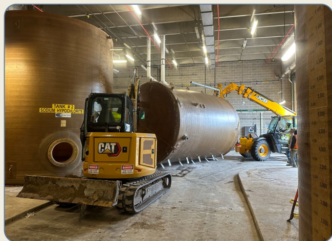
Removal of tanks from chemical feed room for the conversion to gas chlorine
