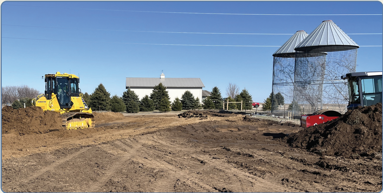
Before the spring blizzard in late March, Rice Lake mobilized equipment, a job trailer and formed up the driveway for the Larchwood pump station site. They will resume construction when conditions allow. This project is part of the expansion to 60 MGD and the cost is being covered by ARPA funding from the State of Iowa.
