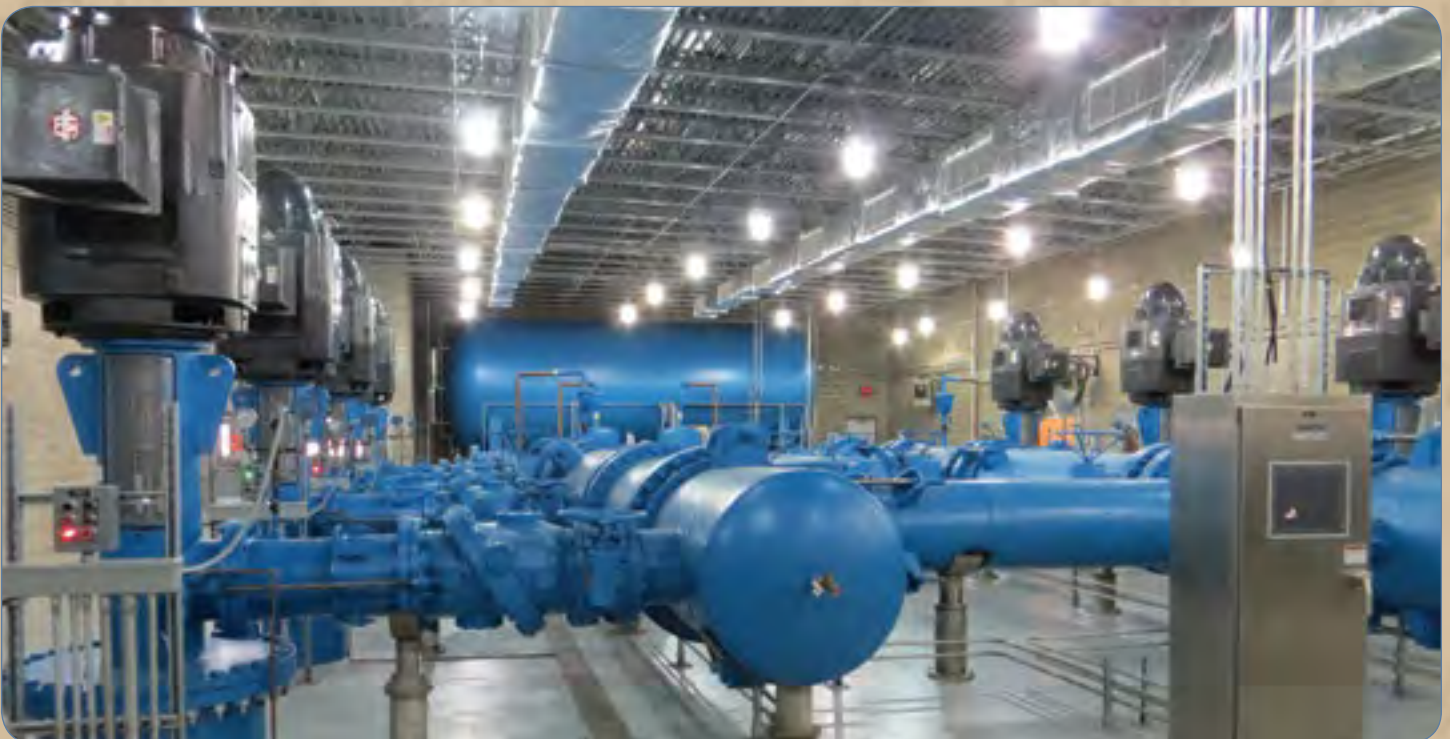
Pump room of the Tea pump station. Eriksen Construction finally reached substantial completion on April 6, close to five months past the deadline. Delays involving the delivery of the eight 350 h.p. high service pumps and the associated control panels were the main reason for the delay.
