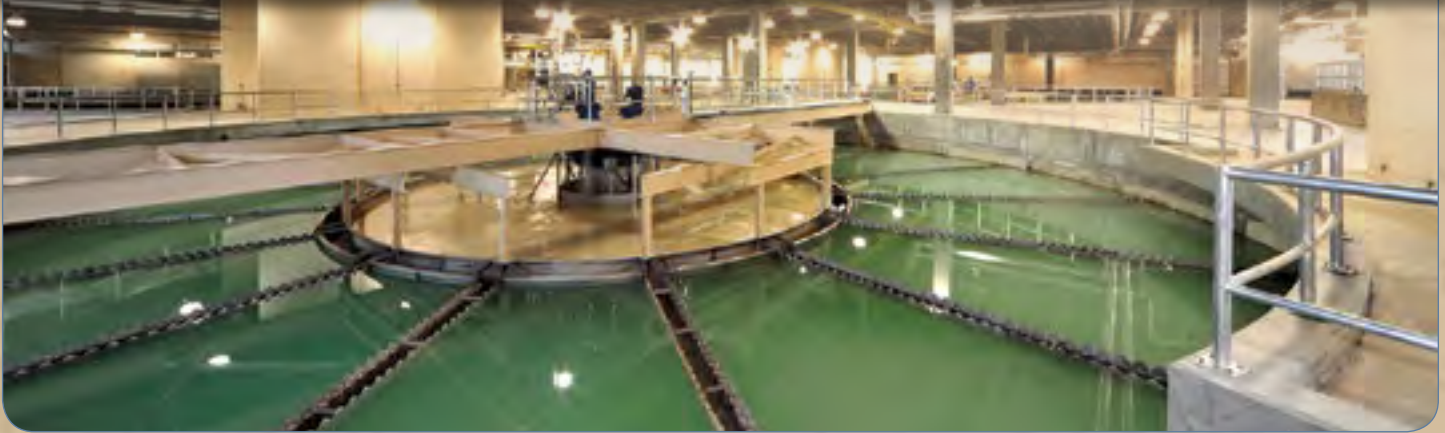
One of four solids contact basins where lime (brown center area) is mixed with the water. The basins are 85' in diameter.
