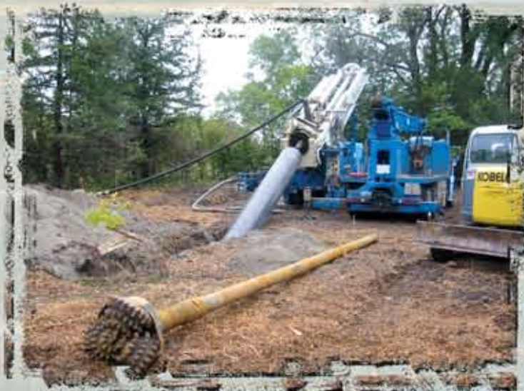
Angle well being drilled at Mulberry Point south of Vermillion, with the 24" drill bit in the foreground.
