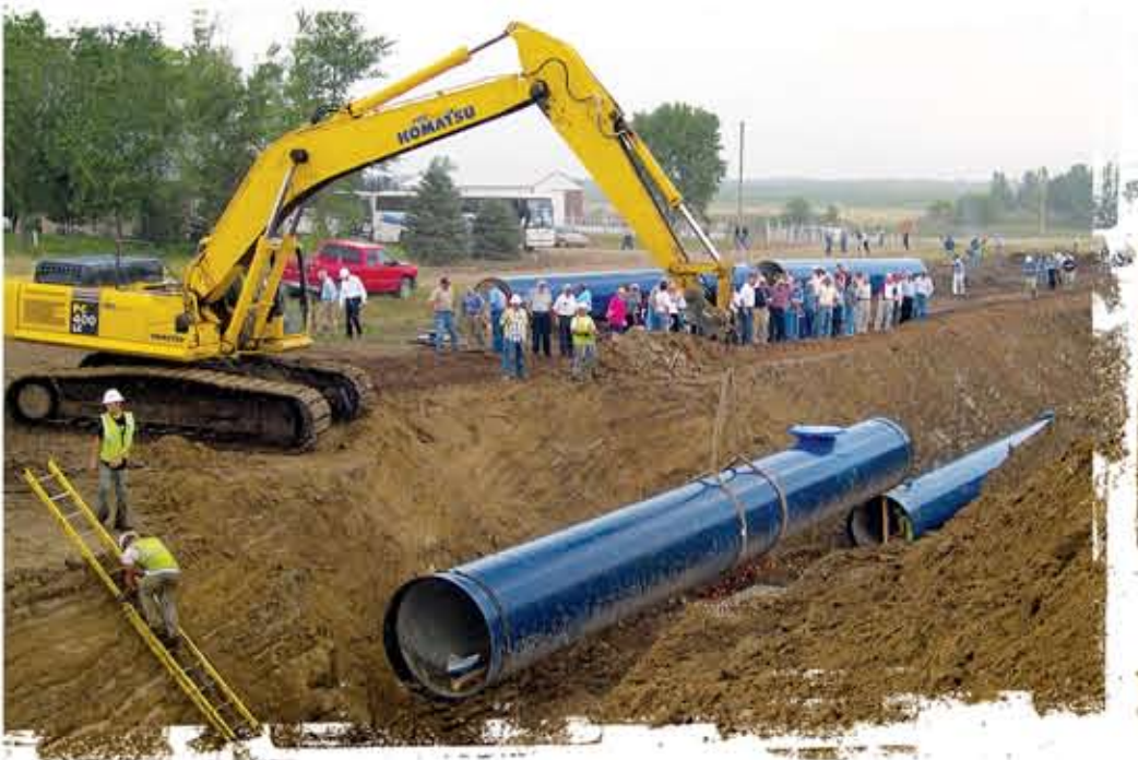
Members watch 54" pipe being installed on Segment 2 of the treated water pipeline near Lennox.
