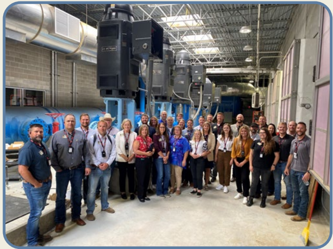
Shown in the high service pump station, Duchscher (far right) on July 24 gave a tour to the SD Agriculture & Rural Leadership class, as well as provided background on the history and future of L&C
