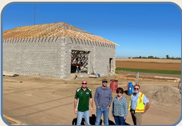
Left to right: Executive Director Troy Larson, Construction Administrator Clint Koehn, Business Manager Lori Seten and Operations Manager Jim Aven check out progress on the Larchwood pump station on September 25
