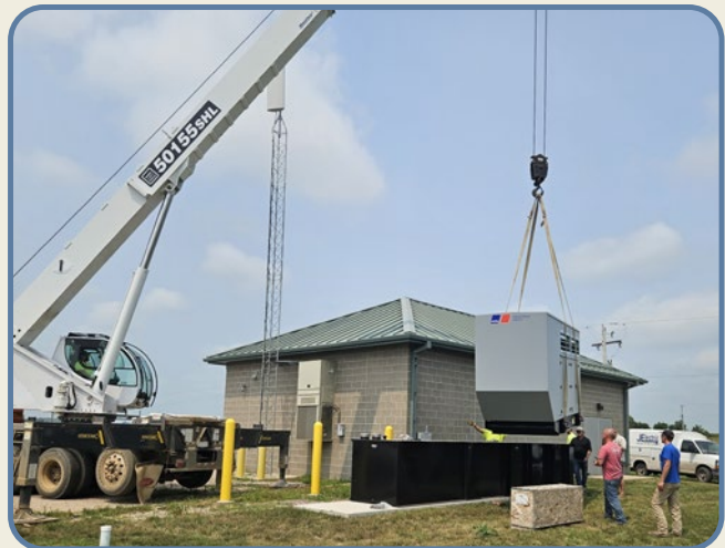
The long-awaited backup generator finally arrived for the Crooks pump station, allowing D.W. Proehl to reach substantial completion on July 26, which was the substantial completion deadline so just in the nick of time!
