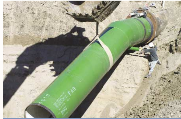
54" diameter pipe angles down after coming through the Highway 50 boring. This is the first section of pipe shown on the front page.
