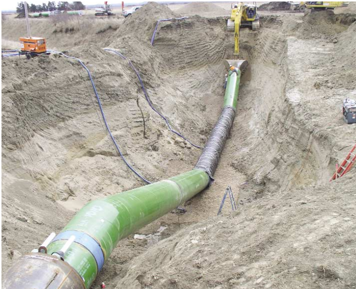
54" diameter pipe on RWP-3 extends from the Hwy 50 boring. The pipe dips to get underneath the Yankton-Clay Drainage Ditch on the south side of the highway.
