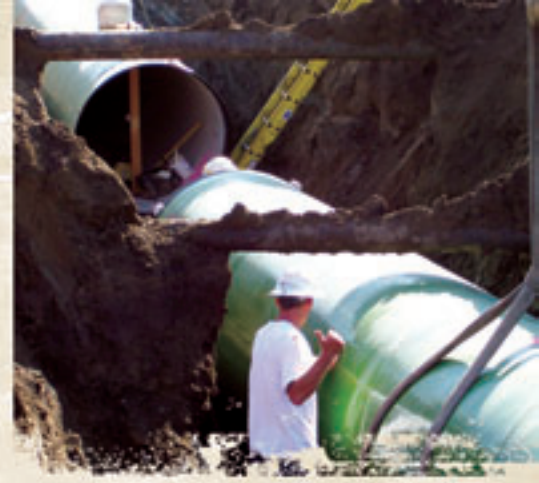
High Country Pipeline installing 54” diameter pipe under two natural gas lines west of Vermillion.
