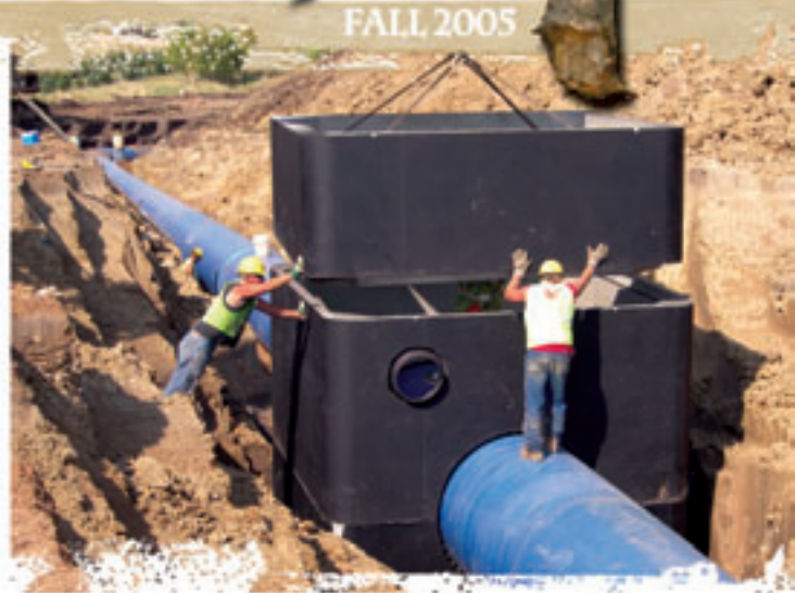
A pre-cast air vacuum vault is lowered into place west of Tea (see air vacuum valve on pg. 6). The diameter of the main trunk line was increased from 48” to 54” to accommodate the additional capacity requested by Sioux Falls.
