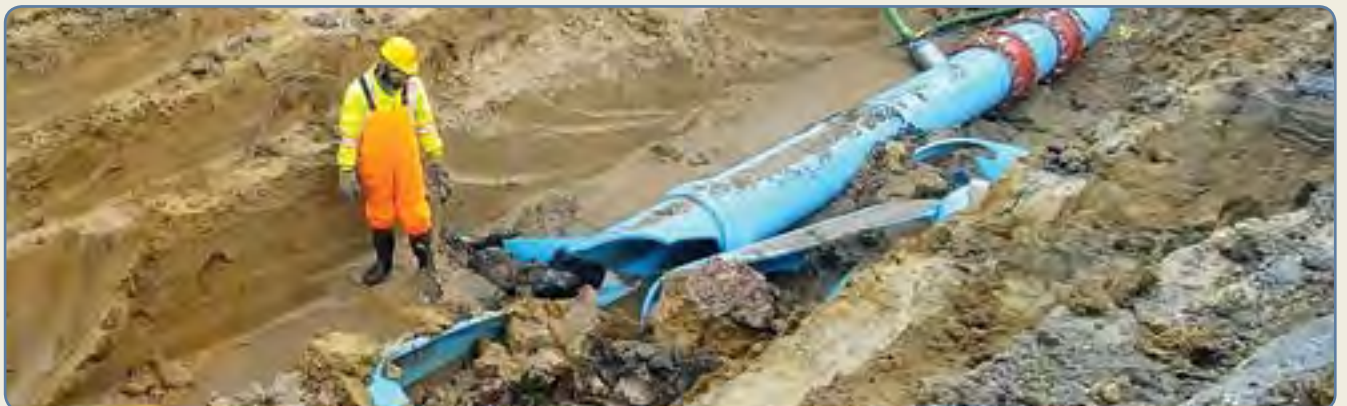
Below: Mistakenly cutting into the pipe while it is still under pressure causes it to burst with explosive force. Fortunately, nobody was injured.
