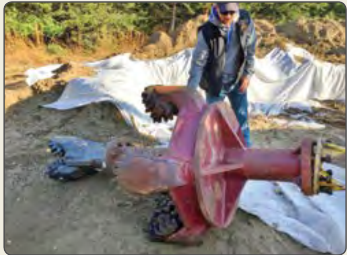
48 inch diameter drill head used to bore 100 feet deep for the replacement well
