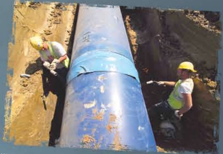
Workers on TWP-5 use blow torches to heat a "shrink wrap" that seals the joints.
