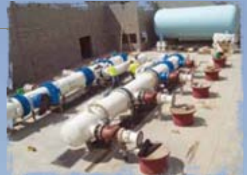
Process piping being installed and painted on the main floor of the pump station, with the surge tank in the background.
