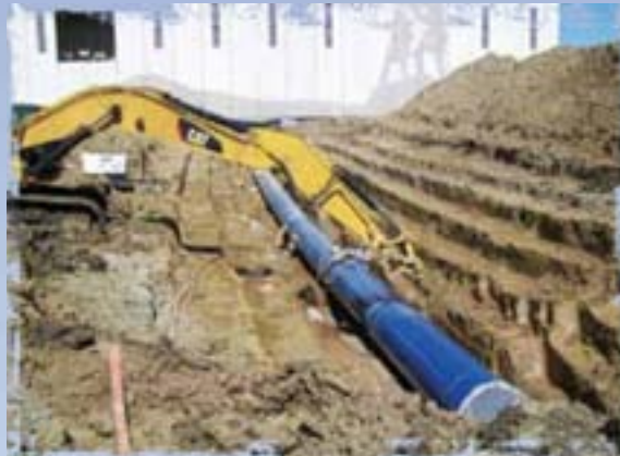
54" raw water pipeline being installed on the south side of the treatment plant. This line will bring untreated water from the wells to the plant.
