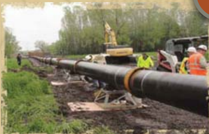
24" ductile iron pipe that was pulled through the directionally drilled bore under the Big Sioux River.
