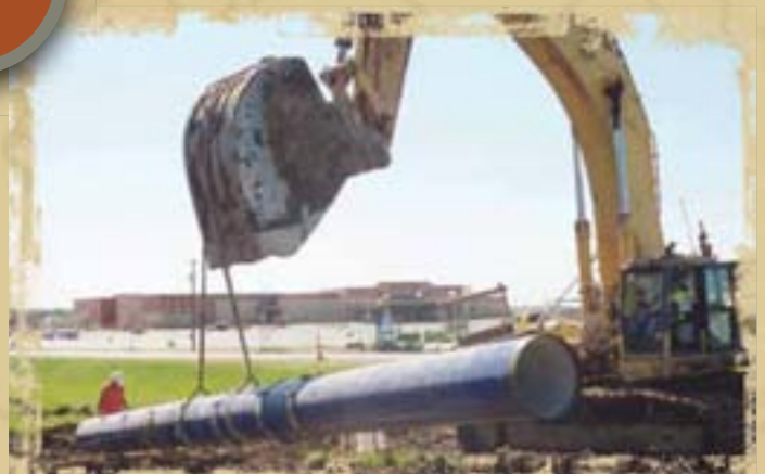
24" pipe being installed on the SD side, with the new casino in the background on the IA side.
