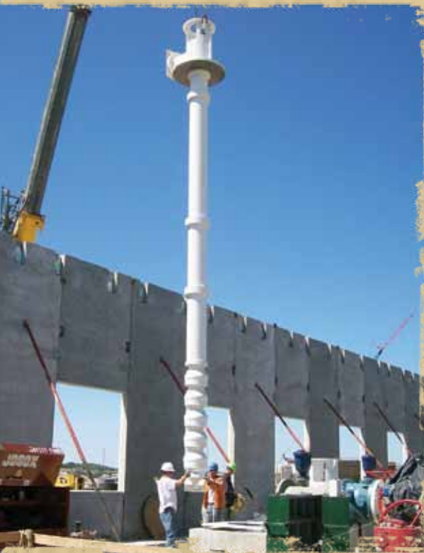
One of four high service pumps being installed in the pump station. Pre-cast wall panels going up in the background.
