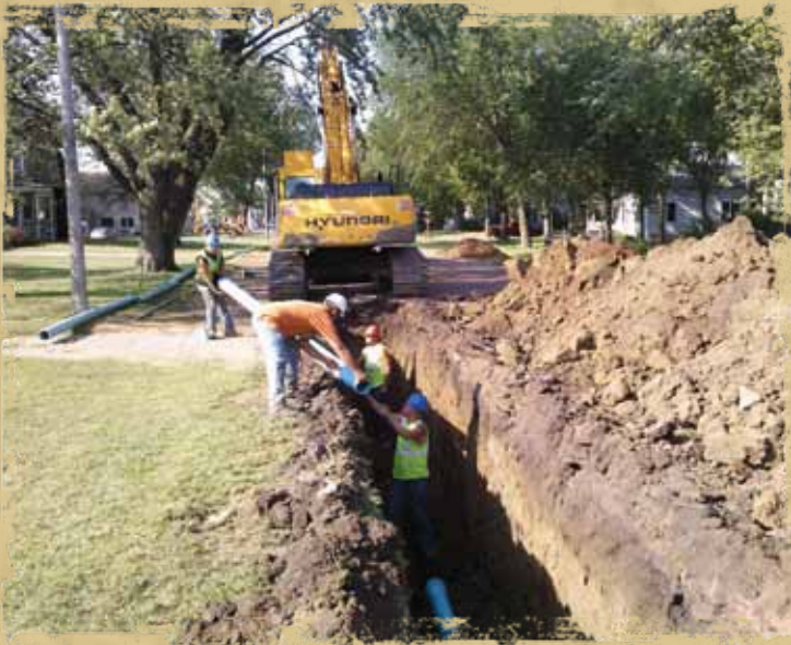
Nitteberg Construction installing 6" PVC pipe in Centerville as they near the end of the service line.
