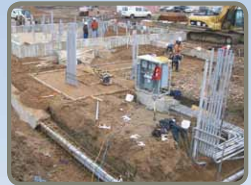
Electrical conduit being installed for the electrical switchgear building (background) and the pads for the backup generators (foreground).
