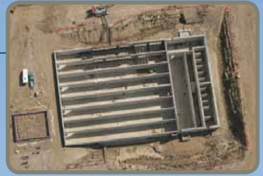
The left side shows the maze of walls for the clearwell portion of the underground reservoir that ensures the first water in from the treatment plant is the first out. The wet well portion (pump station will sit on top) is on the right. To the left of the reservoir are the footings for the electrical switchgear building.
