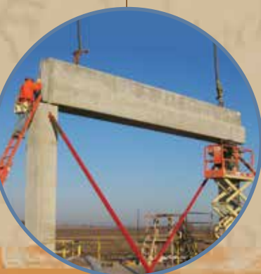
Columns and beams being set for the main floor walls of the solids contact basin area.
