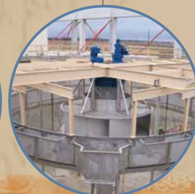
Mixing equipment being placed in one of the four solid contact basins.
