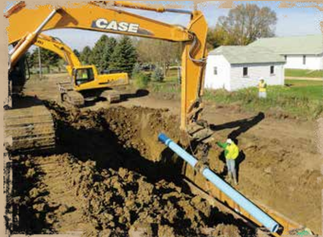
10" PVC pipe being installed on the south side of the rural Germantown Presbyterian Church near Parker.
