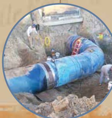
The final 54” tie-in to connect the underground reservoir and pump station with the main trunk line.
