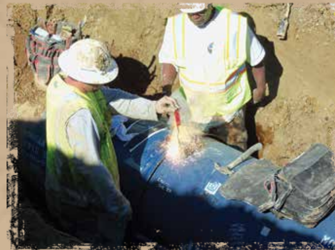
"Cadweld" charges are ignited to weld the joint bonds that connect the pipes. A low voltage electrical current helps protect the pipe from corrosion (cathodic protection system).
