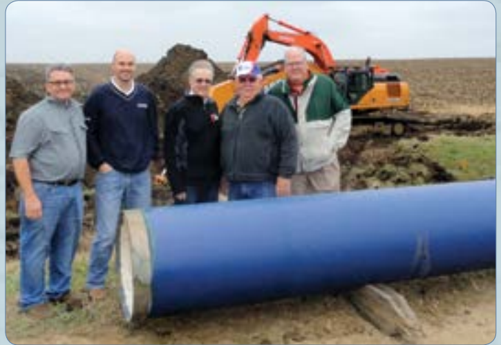
Construction Administrator Dan Zulkosky, Executive Director Troy Larson, Luverne Councilman Kevin Aaker, Chairman Red Arndt & Luverne City Administrator John Call signed the last piece of pipe
