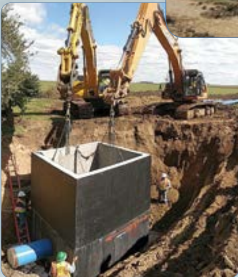
Below: Isolation valve vault
