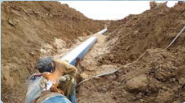
Most joints are just pushed together but they are welded where the pressure is higher or a leak is fixed
