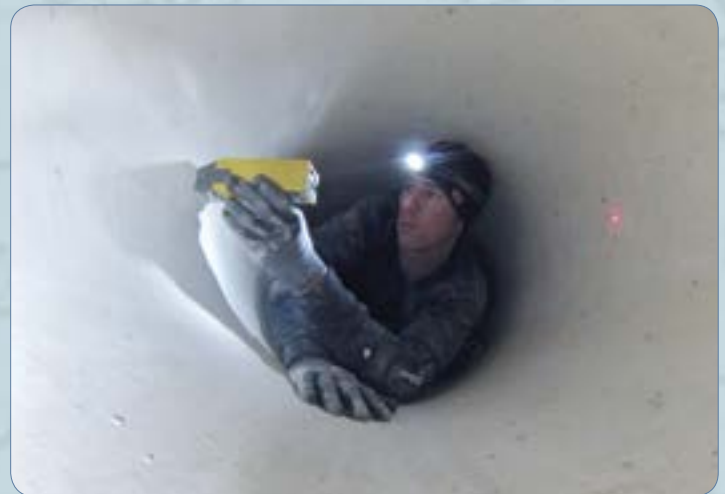
Banner's Clint Koehn crawled the 12.5 miles of 24 inch pipe to inspect the joint grouting and deflection (roundness). Tight squeeze!
