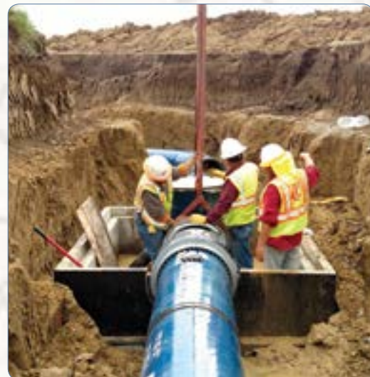
Isolation valve vault
