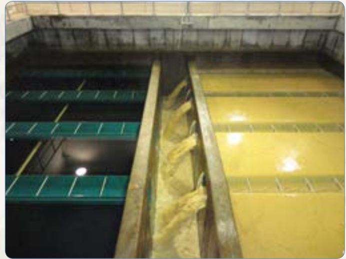
The left side of this filter has been backwashed and the right side is being backwashed. With the increased demands each of the eight filters are being backwashed about every two weeks.
